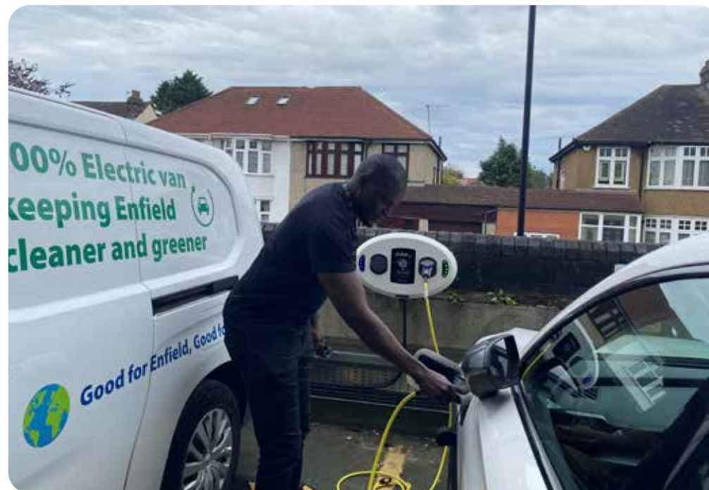
Electric vehicle charging point
